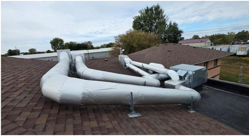
Energy Recovery Ventilation (ERV) System installed on rooftop.
